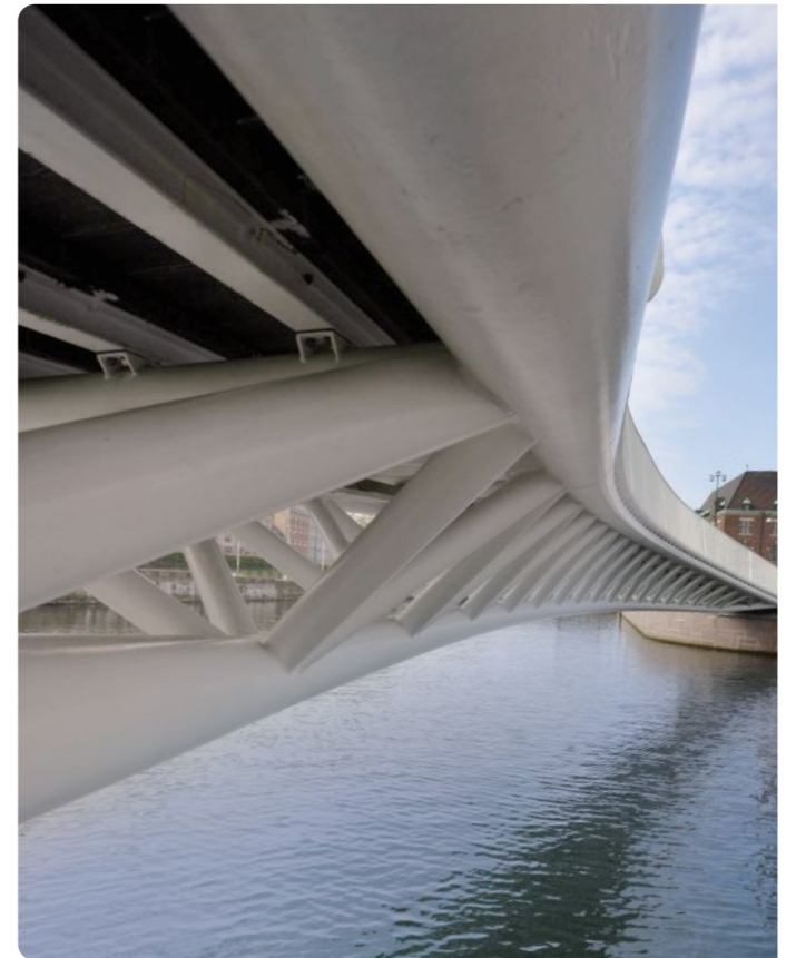
During the structural design of the pedestrian bridge at Baggers Plats in Malmö, it became obvious that it would require a TMD, as the lowest vertical was calculated to 1.85 Hz.
